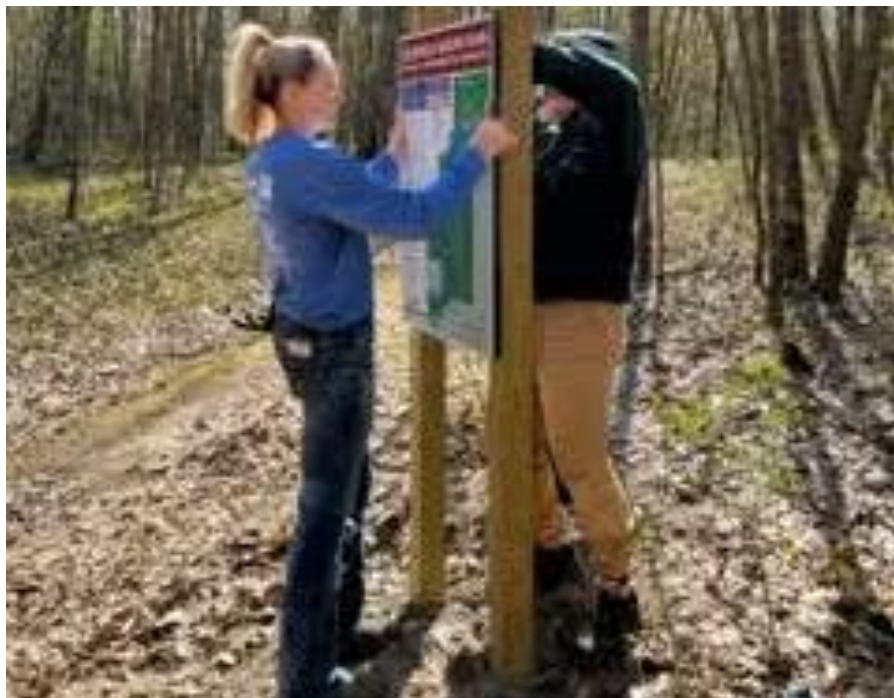
Mt. Pleasant Rotary Club helped Eagle Scout Eli Bucilli and local Boy Scouts install wayfinding signs at Deerfield Park to assist park visitors while they explore the trails
